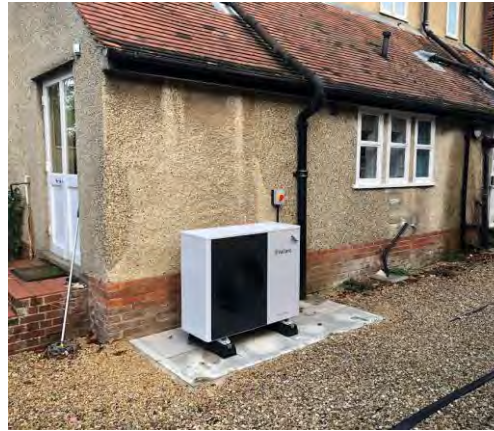
Domestic 7kW unit
